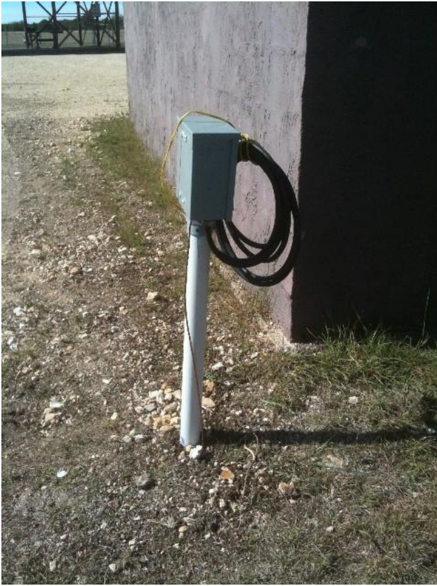
Generator Connection Point
