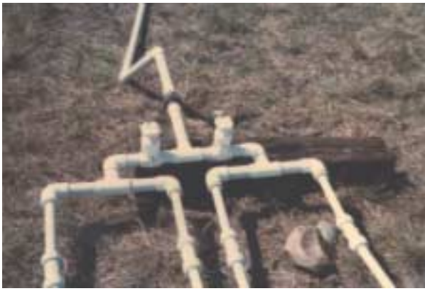
Head manifold splitting into 4 lines
