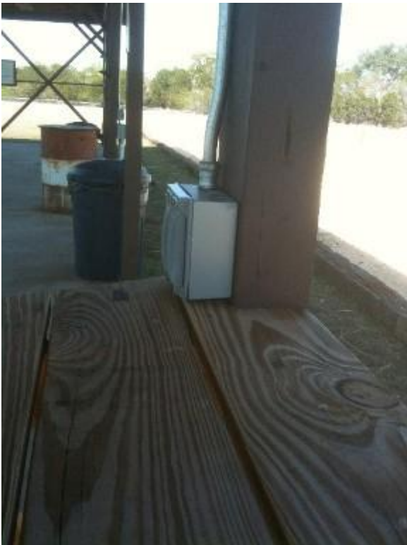
Charging Station Outlet
